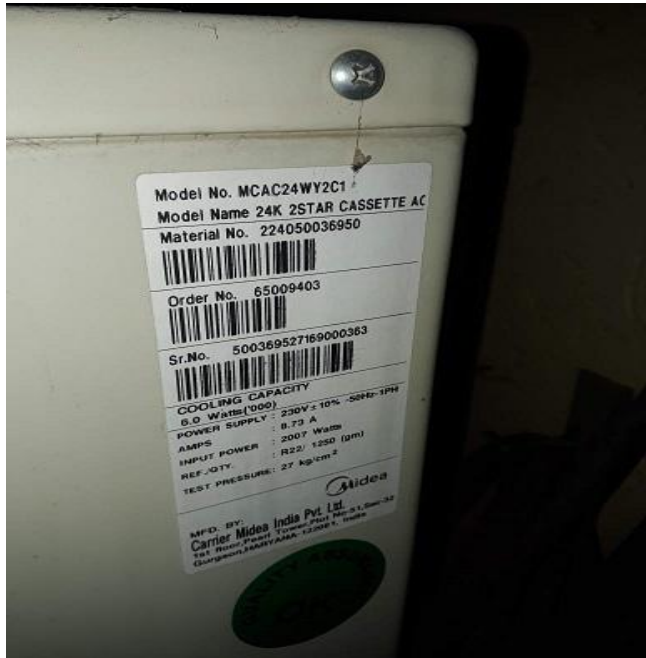
AC UNIT OUT DOOR UNIT NAME PLATE DETAILS
